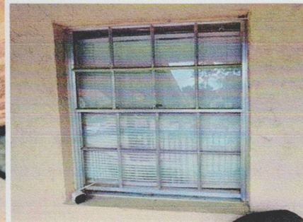
Unprotected glazed opening
