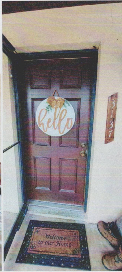
Unprotected non-glazed entry door
